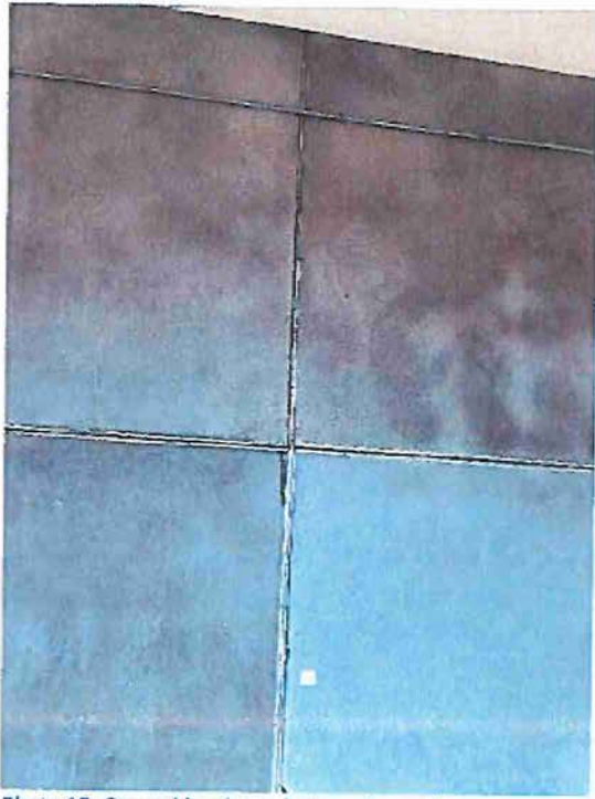
Photo 15: Ground level, cracks in wall panel.
