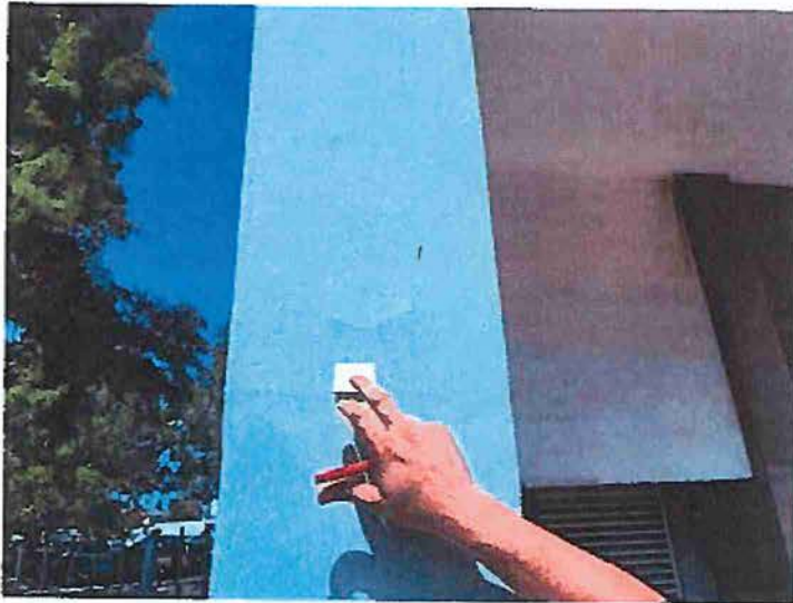
Photo 22: Ground level, Column O-16, spalling skim coat.
