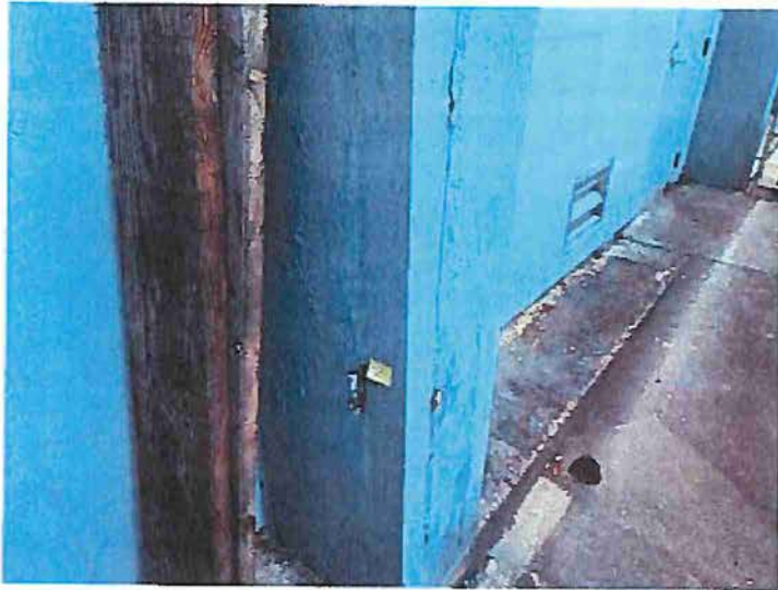
Photo 26: Ground level, column L-2, spalling concrete.
