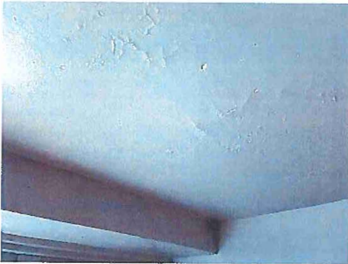
Photo 29: Interior room, water infiltration, flaking paint.
