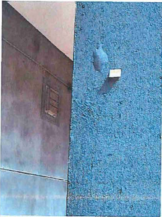
Photo 13: Ground level column, O-5, water infiltration.
