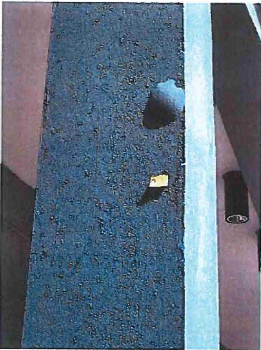
Photo 12: Ground level column, O-7, water infiltration.
