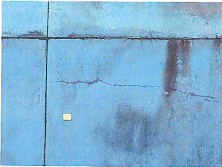
Photo 18: Ground level, crack in wall panel
