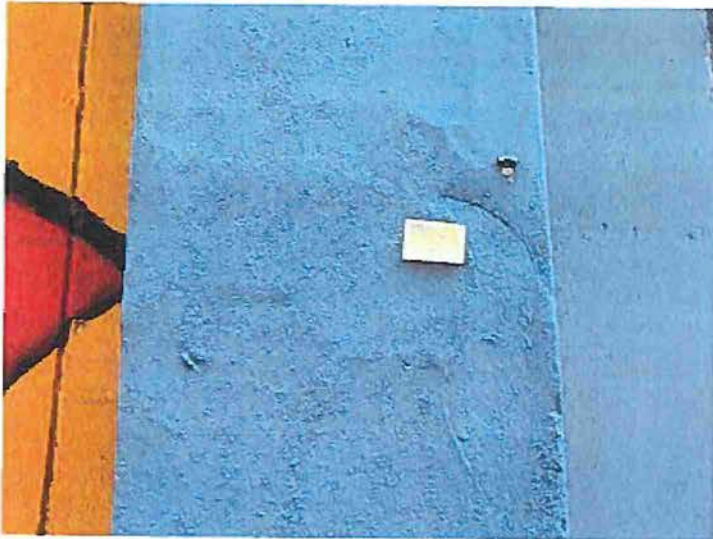
Photo 24: Ground level, Column L-23, old patch water infiltration.
