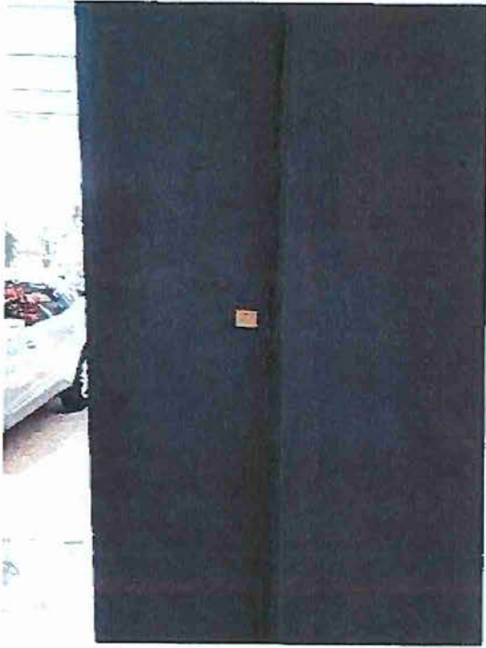
Photo 21: Ground level, column O-16, joint sealant cracked.
