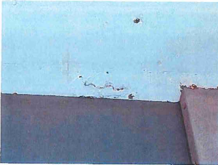
Photo 20: round level spall in soffit panel.
