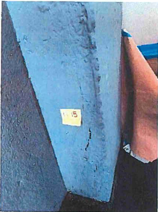
Photo 10: Roof level column, N-15, cracked.
