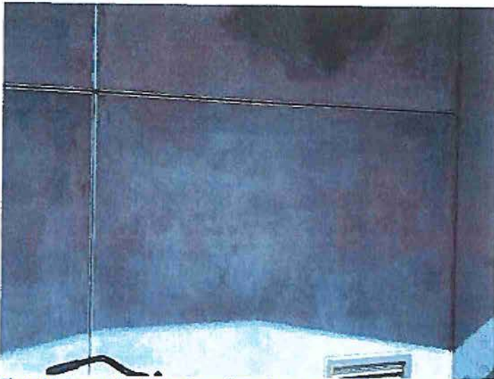
Photo 14: Ground Level, exterior wall panel cracks at joint.
