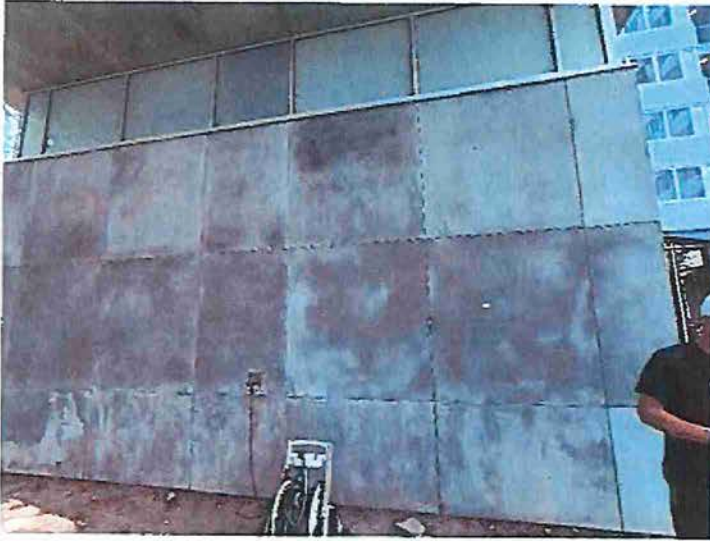
Photo 19: Ground level, crack in wall panels.
