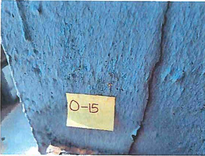
Photo 7: Roof level column, O-15, cracked.
