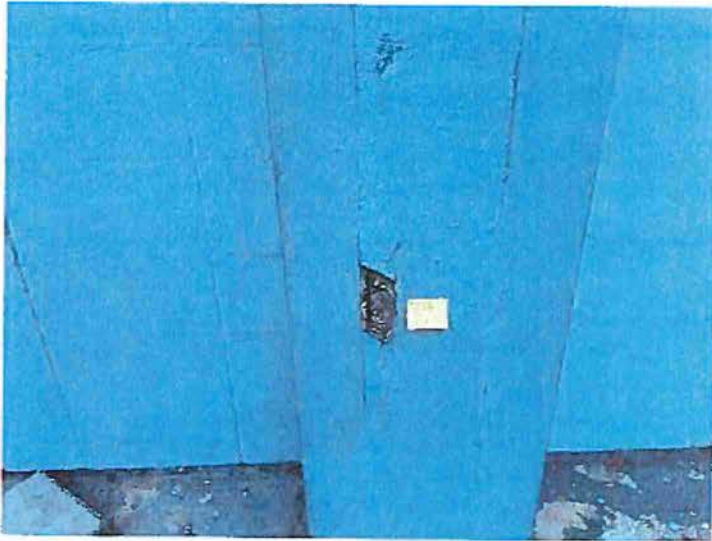
Photo 25: Ground level, column L-6, spall.
