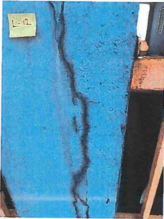
Photo 5: Roof level column, L-12, cracked.
